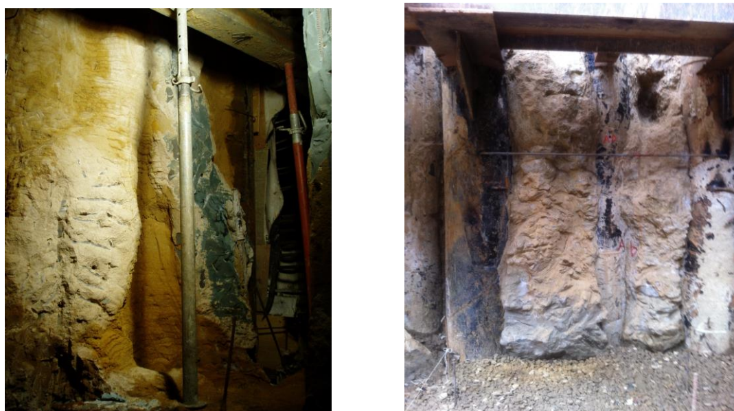
Figure 1. The view of the grouted soil sections using impregnation (left) and jet (right) cement grouting
